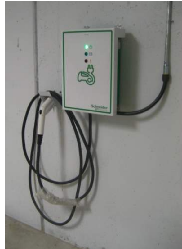
Wall Mounted Stations
